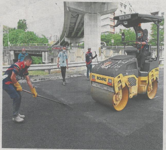
DBKL task force repairing potholes in Jalan Sri Permaisuri, Kuala Lumpur. — Filepic
