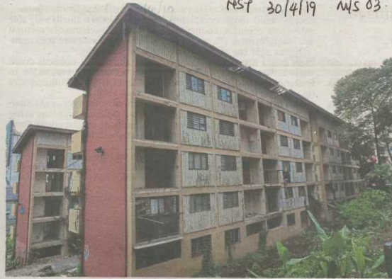
Residents of Block F of Taman Keramat Permai flats in Ampang Jaya, Selangor, were evacuated following the discovery of cracks at the block on Friday. PIC BY ASYRAF HAMZAH
