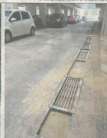
Drains inside the flats clogged with dried mud.
