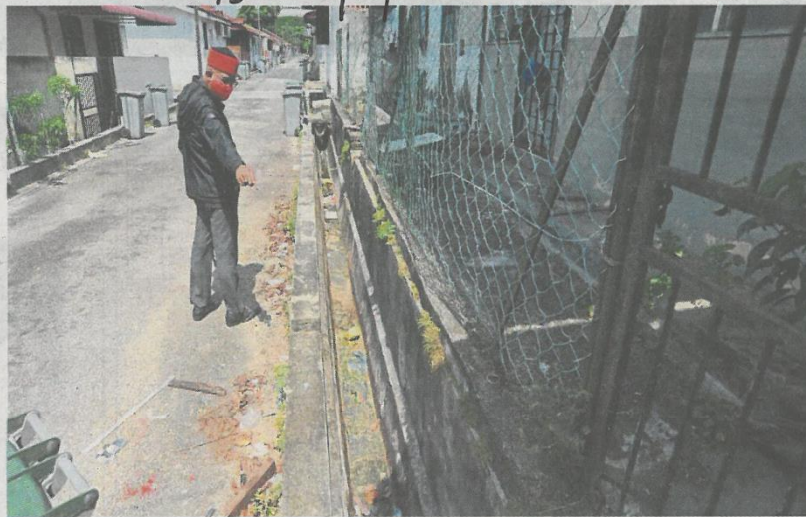
Salahuddin showing a rubbish-clogged drain along Jalan Jelatang 27 in Taman Megah Ria, Johor Baru.
