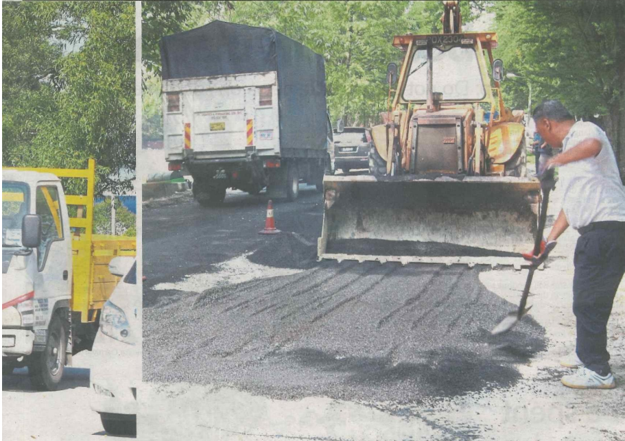
Road tarring works along Jalan 225 in Section 51A. Izham hopes that the problem of who is responsible for a particular road will be resolved soon. — Filepic
