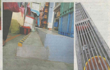
Customers say the split level at Pasar Pandan Jaya makes it dangerous to walk.
