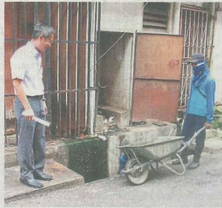
Lai inspecting the cleaning of a drain by KDEBWM workers in Taman Muda.
