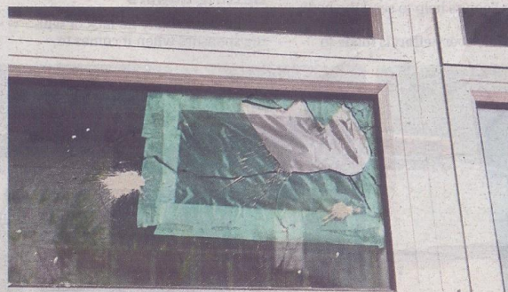
A kitchen window of a resident in Taman Bukit Segar Jaya 1, Cheras, which was damaged after a cement bucket fell from a luxury condominium construction site.
