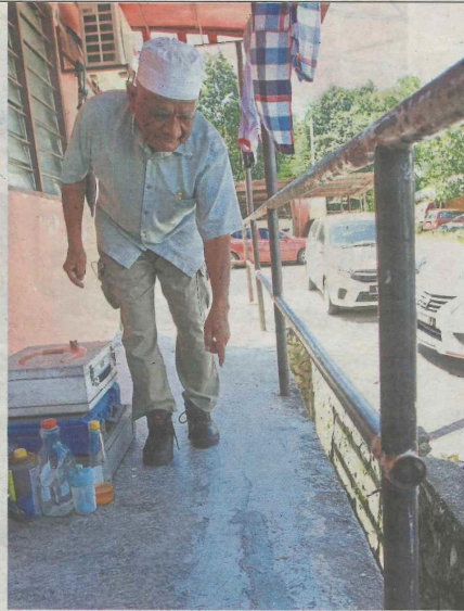
Mohammad Saidin showing cracks that he claims to have reappeared on the floor after the repair work. — Photos: LOW LAY PHON/The Star
