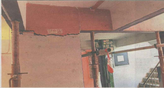
Cracks are seen on walls and iron beams have been placed near the staircase (right) to support the structure.
