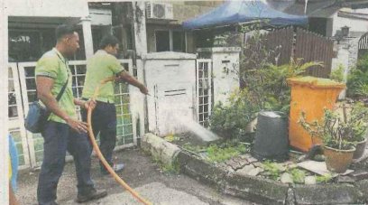
MBSA contractors using water jets to clear the clogged drains in Taman Sri Muda.
