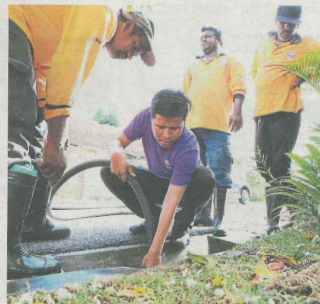
Ameer (centre in purple) using a high pressured water hose to push out silt and dried leaves beneath the concrete culvert at Jalan 10/3 in Section 10, Petaling Jaya.
