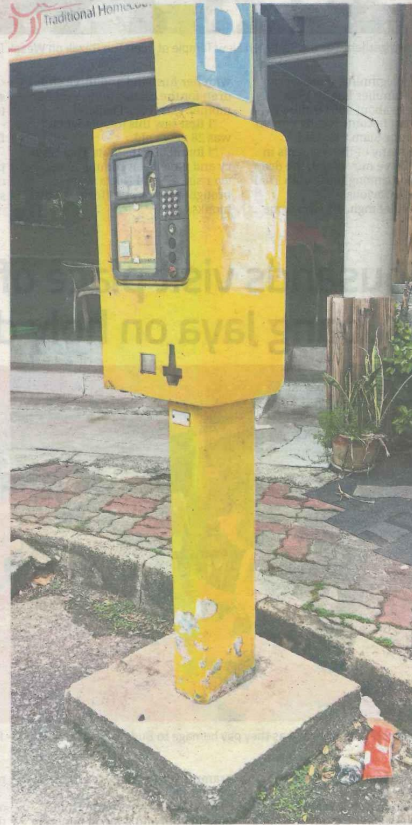
There are over 700 parking machines in the city to cater for about 21,000 parking bays and today over 50% of them are faulty.
