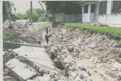
The debris of a collapsed retention wall of a home in Taman Ukay Heights following a mudflow on Nov 11. — Filepic
