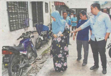
Suzana (left) and Rosdi (centre) inspecting the broken drains and gaps formed beneath one of the buildings. — Photos: ANIS ABDULLAH/The Star
