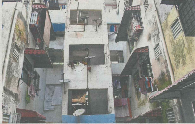
Signs of water damage from leaky pipes visible on the walls of the Seri Impian flats.
