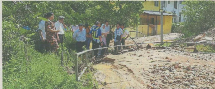
Zuraida (in headscarf) ordered the highway concessionaire to start mitigation works to prevent a recurrence of the mud flood after her site visit to Sierra Ukay.
